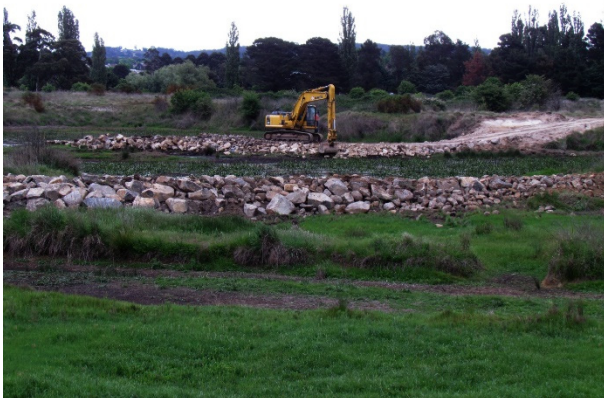
Creating a berm wall in the Mulwarree River wetlands region of Goulburn (2011)
