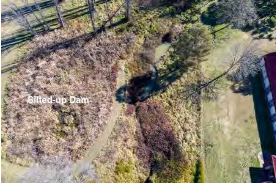
Figure 7: Aerial view of the silted-up dam adjacent to Black Gully. Photo: Terry Cooke.
